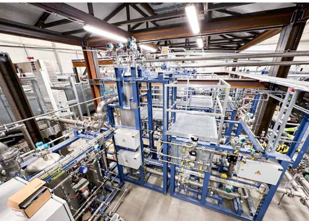
Fig. 2: OffgridWind system (inside) in Floe, Denmark [Source: Thomas Schwabe, Siemens Gamesa, Leitprojekt H 2 Mare]
