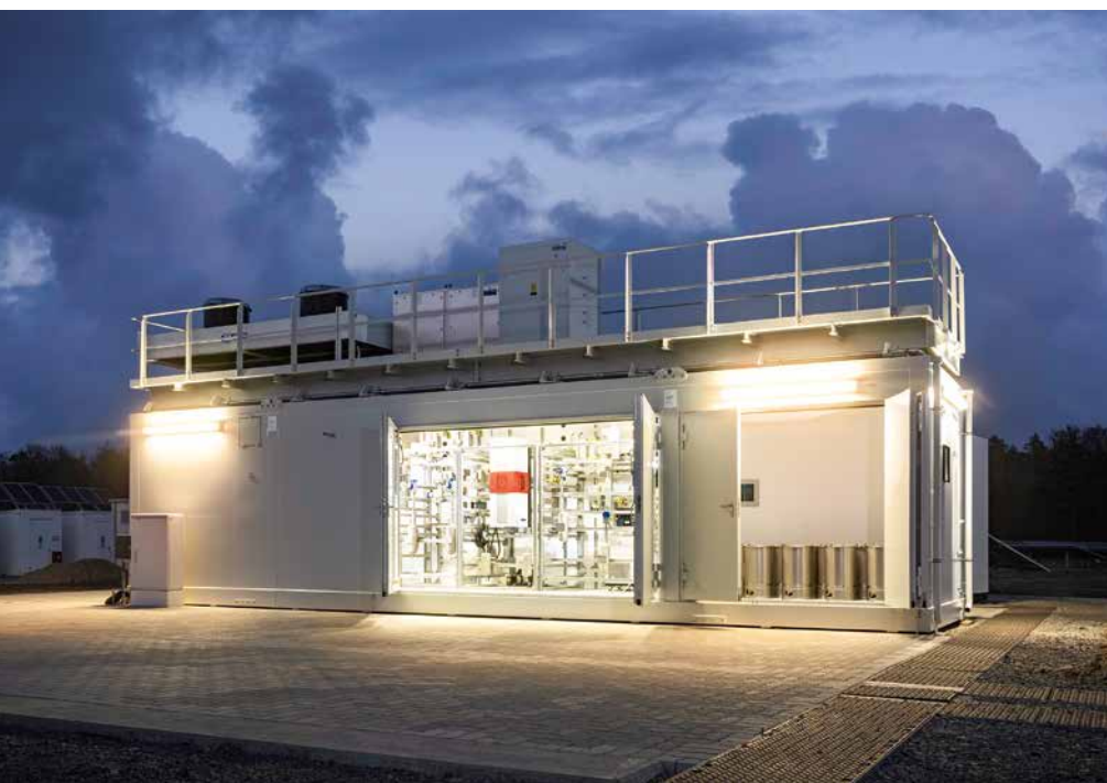
Fig. 1: Power-to-X containerized system for offshore use [Source: KIT]
