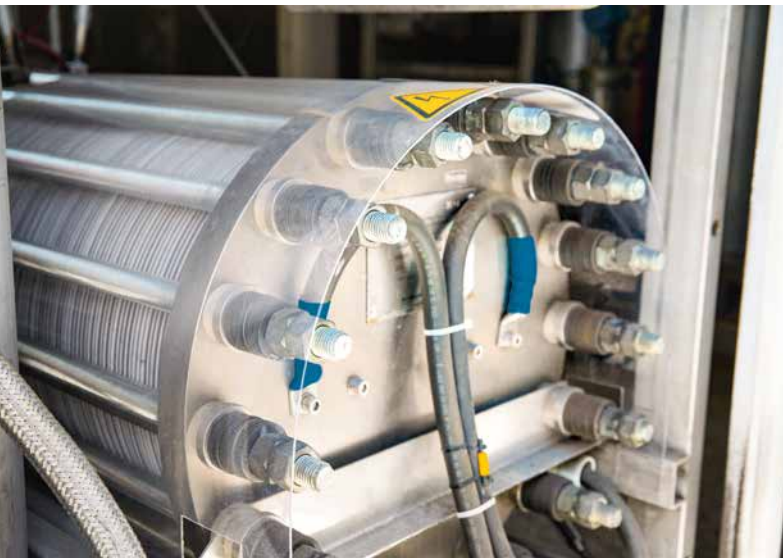
Fig. 3: In hydrogen applications, the quick detection of gas leaks is particularly important [Source: Piltz]
